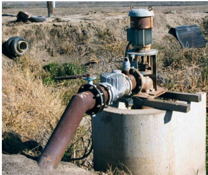
Figure 7. Control (butterfly) valve, air-vacuum relief valve, and check valve located downstream of tailwater return pump. Photo: Lawrence J. Schwankl.
